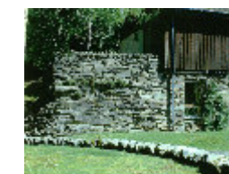
Surviving fabric at the West end of mill 5, rebuilt when Lodge 16 was erected.
